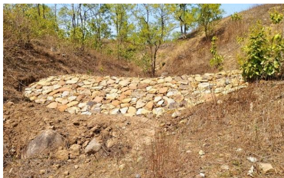
Image 6-20: Loose boulder / Gabion Check Dams
