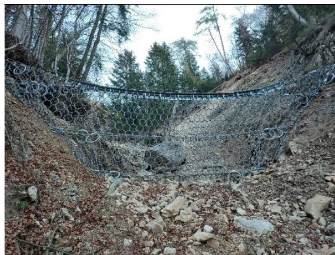
Figure 6-1: Flexible Rockfall Barrier
